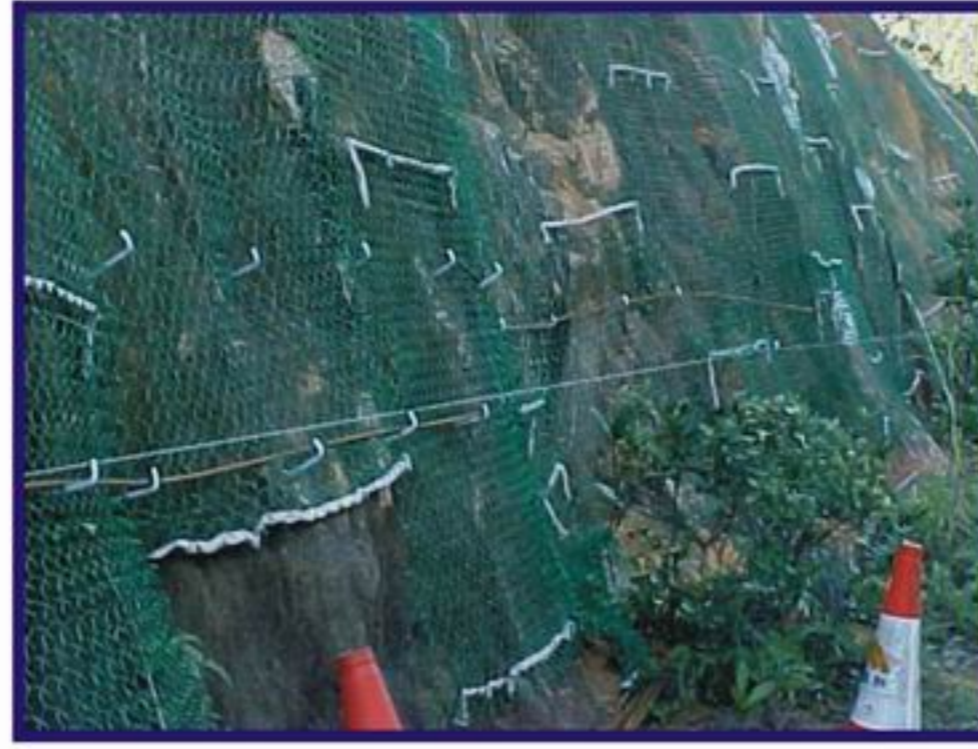
2. Fixing turf reinforcement mat with fertilizer strip by using mild steel bar
